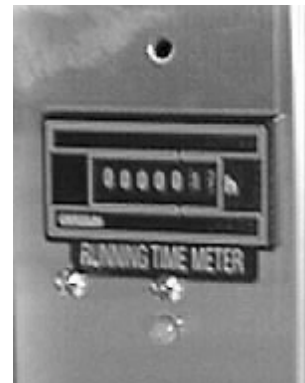
Running time meter with lamp LED indicator.
